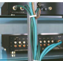
Kabelmanagement Cable Management
